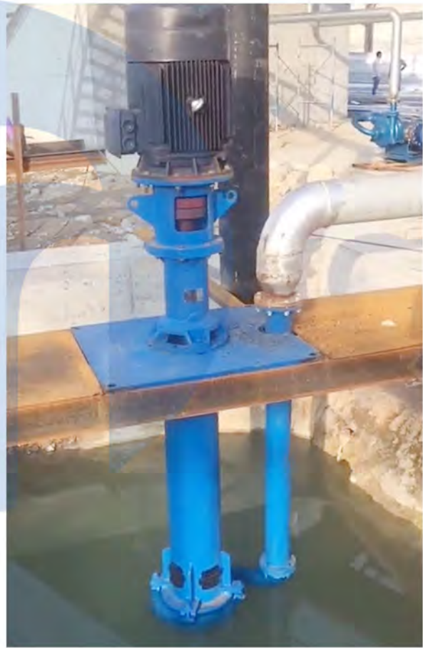
SP pump are used in Wastewater sump, China
